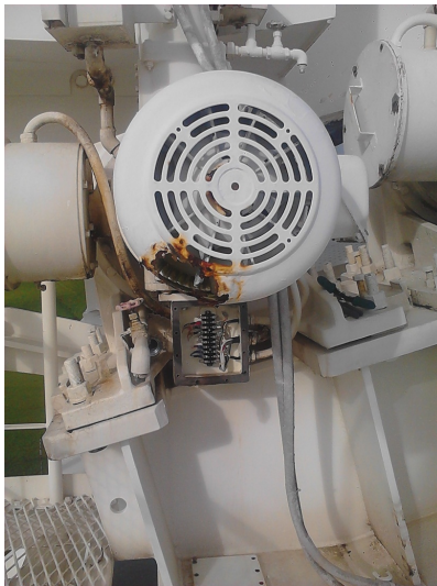
Figure 4. The state of the old motors was very poor and where considered a safety issue.
