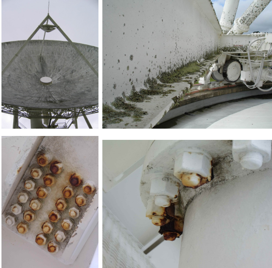
Figure 6. Photos of the 30-m antenna (after cleaning). Images courtesy of Stuart Weston
